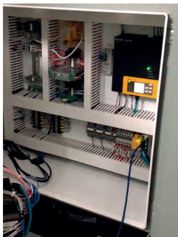
Top right corner shows NGRM700 backplate mount neutral grounding resistor monitor
