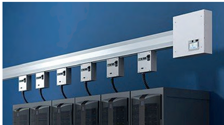
Figure 2: Starline power busway
