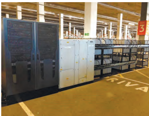
Bender UK supplying 600 kVA modular UPS critical power infrastructure to NHS Nightingale Hospital, Excel center, London
