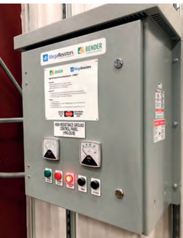
Bender Series 1 Wall Mounted High Resistance grounding package protecting the generators
