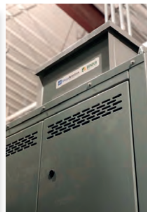
Bender/Megaresistor Neutral Grounding Resistor mounted above switchgear
