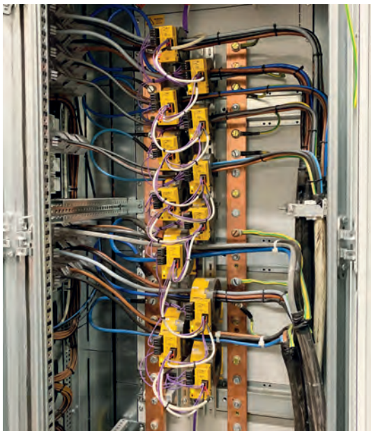
SensorPro residual current monitoring with RCMB301 modules at the outlets of the main distribution
