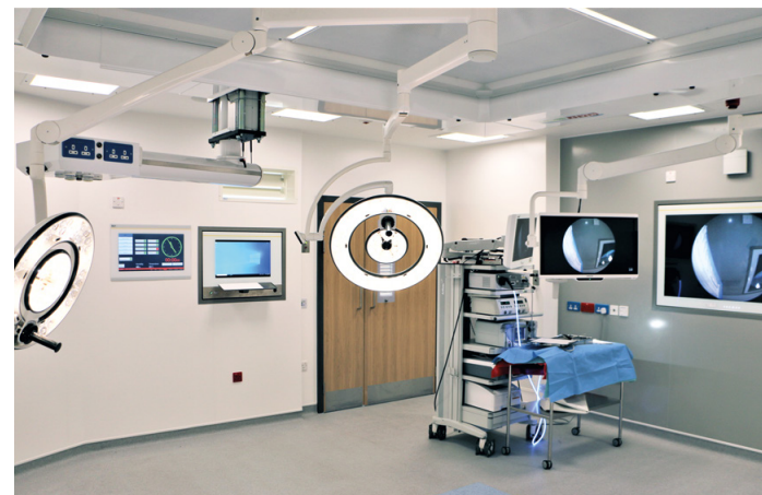
Newly installed theatre at the Elective Orthopaedic Centre (SWLEOC), Epsom Hospital, UK
